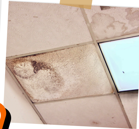
Replace ceiling tiles
